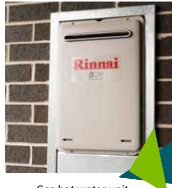
Gas hot water unit.
