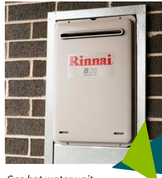
Gas hot water unit.
