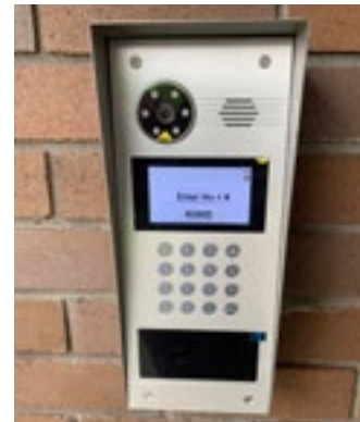
Video intercom panel at the entrance to building
